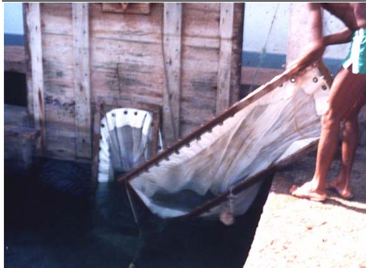
Figure 4.5.14. Installation of filter nets at the sluice gate for Artemia biomass harvesting in solar saltworks.
